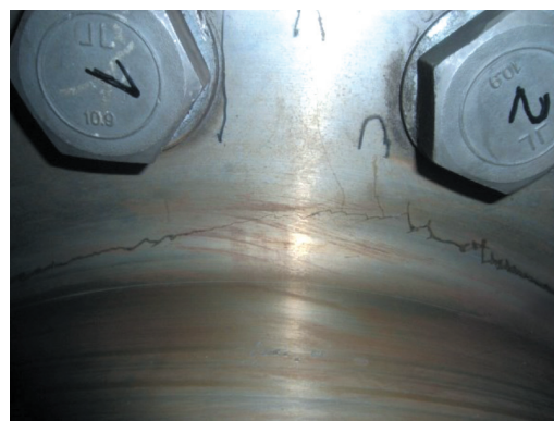
Fig. 3. Cracks on circumference and radial cracks [1]
